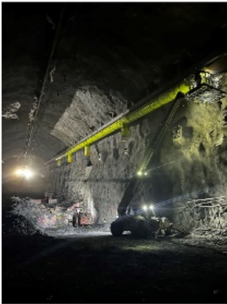
North Cavern (4850-33) adjusting ventilation
